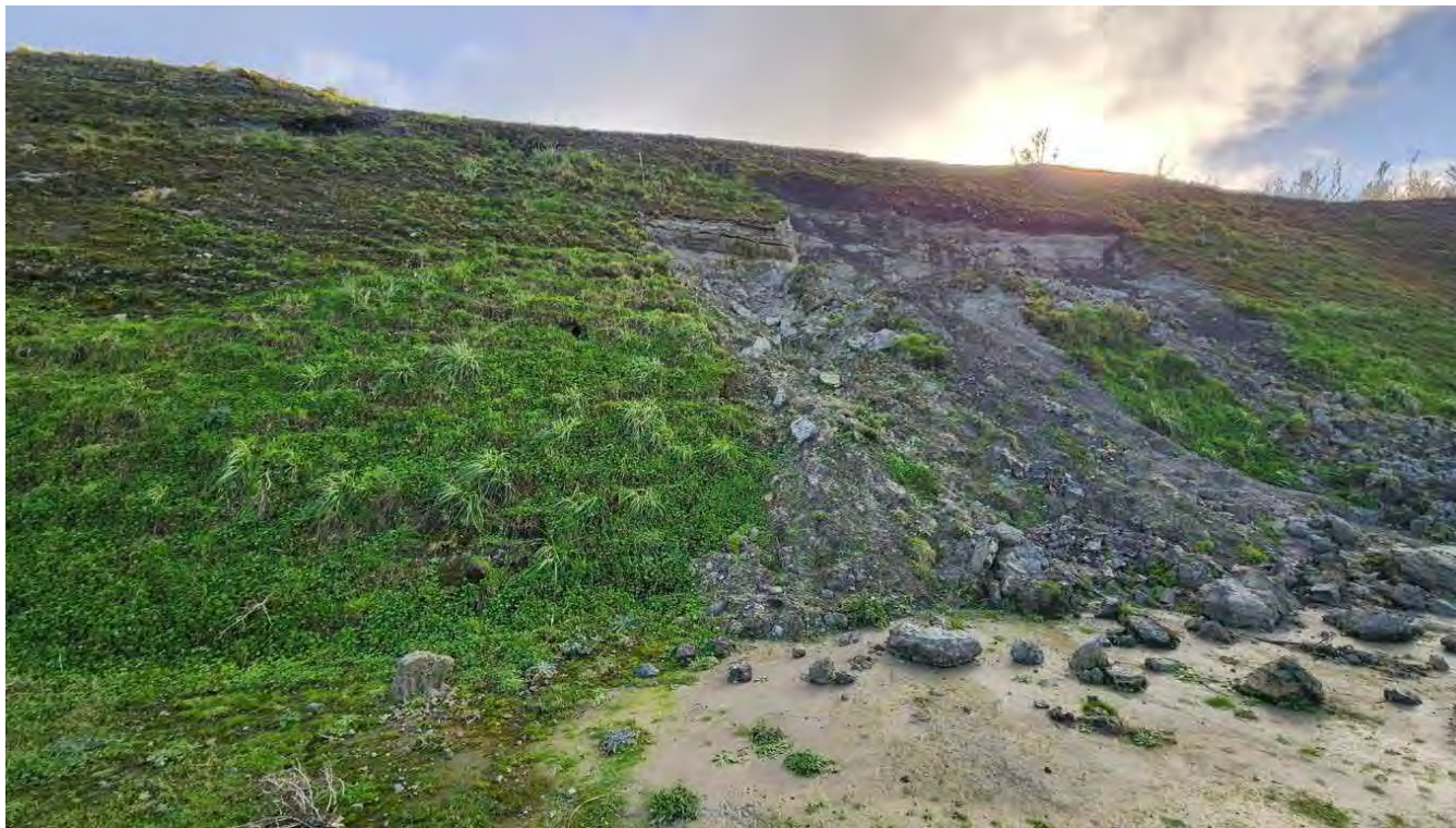
BQ05: Localised batter failure in historic process water fines.
