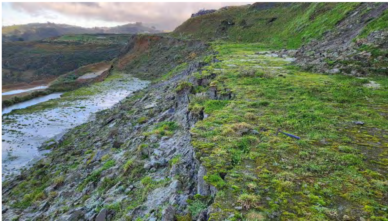
BQ04: Degraded process fines batter where surface water is uncontrolled.
