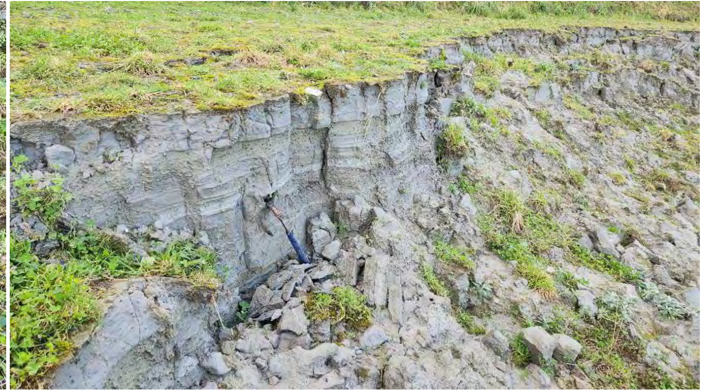
BQ02: Crest of degraded batter with no surface water control.
