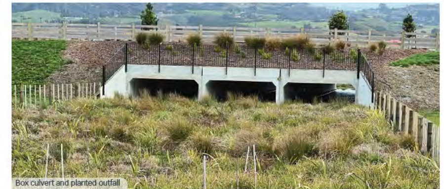
Box culvert and planted outfall Image Clevedon development Auckland
