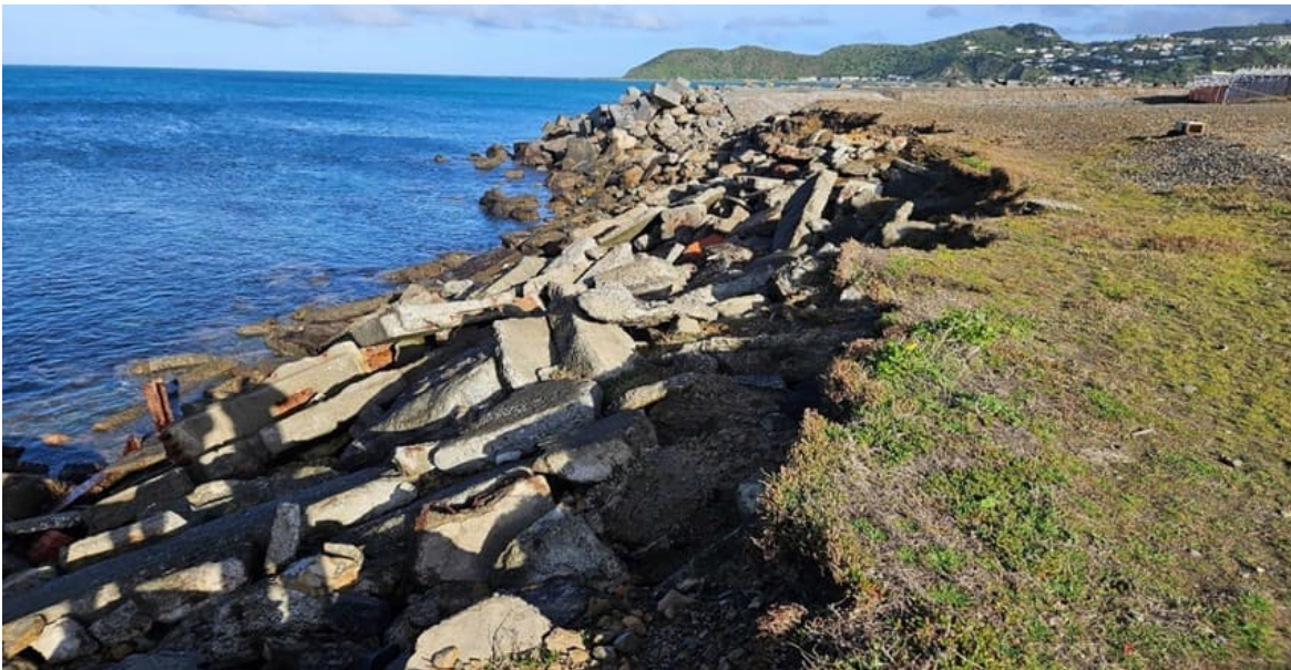
Fig. 4.6. View of the informal eastern area seawall (Construction Area D), looking westward towards the Southern Seawall.
