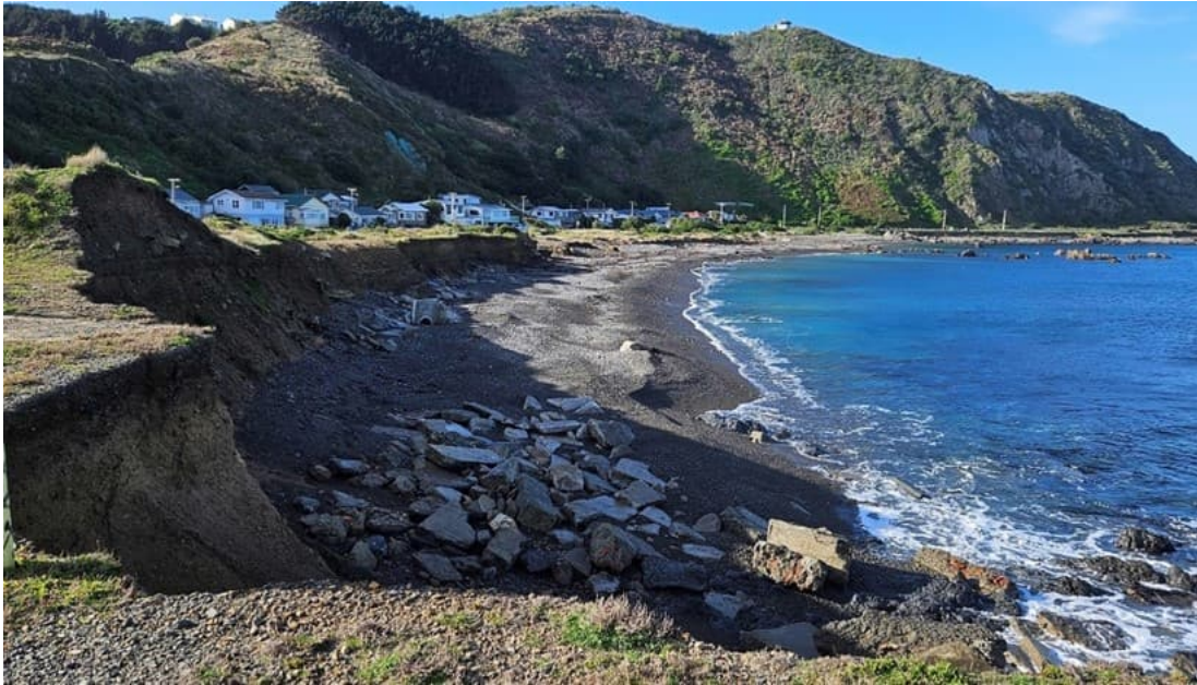
Fig. 4.8. View of the eroding earth bank (Construction Area F), looking eastwards from the eastern end of the informal seawall.
