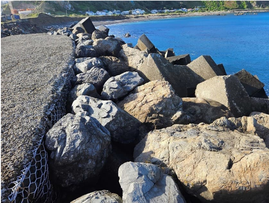
Fig. 4.7. View of the eastern end of the Southern Seawall (Construction Area C), looking eastwards.
