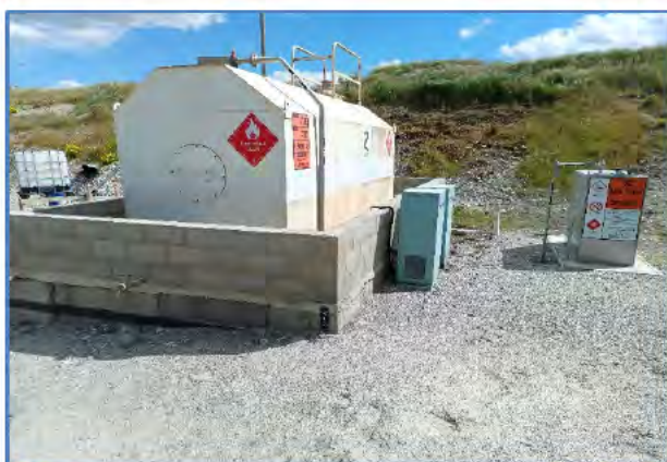
Photo 1: Above-ground diesel storage tank at the asphalt plant.
