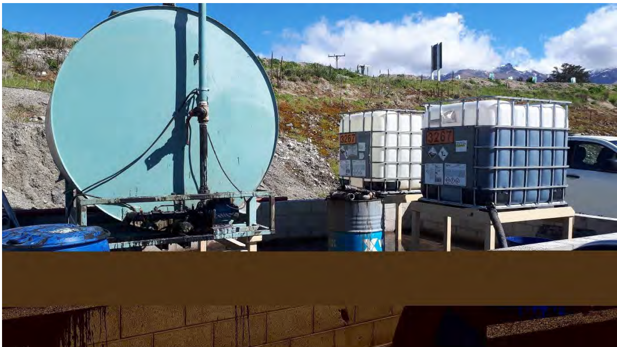
Figure 10: Bitumen storage at the asphalt plant.
