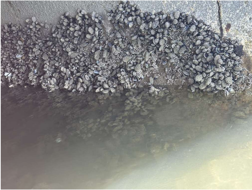
Figure 7 - Mussel beds lining the inner barrel of the Evans Bay stormwater outfall. Photo taken September 2025
