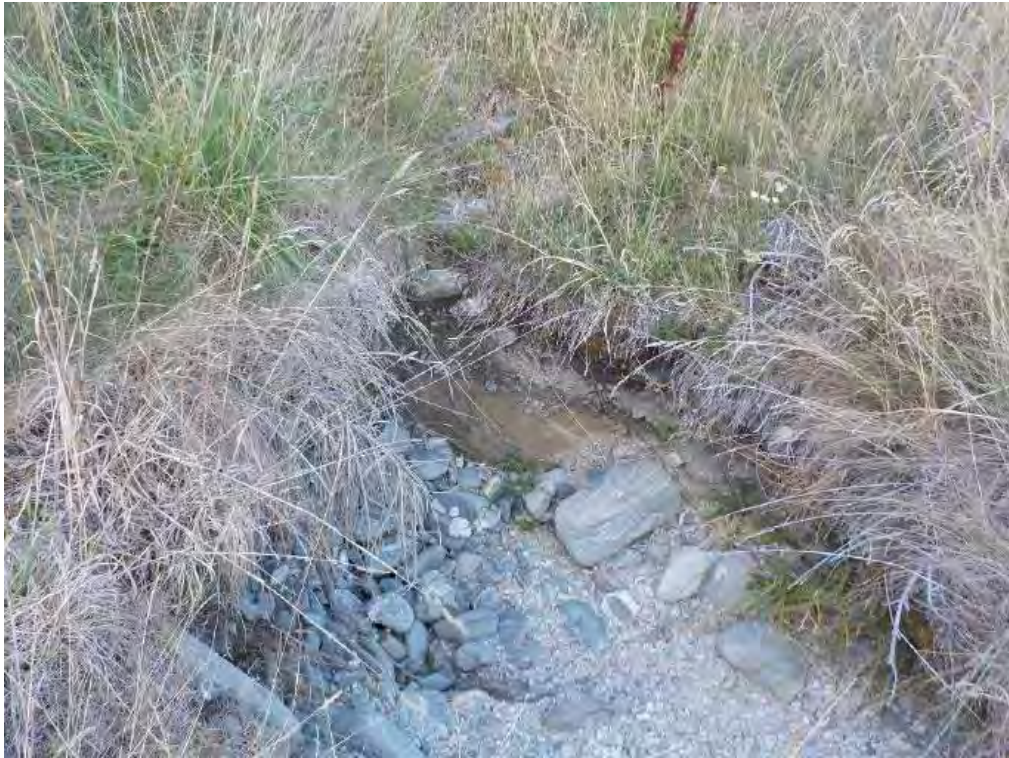
Figure 10: Scour pool in Stream Course 2.
