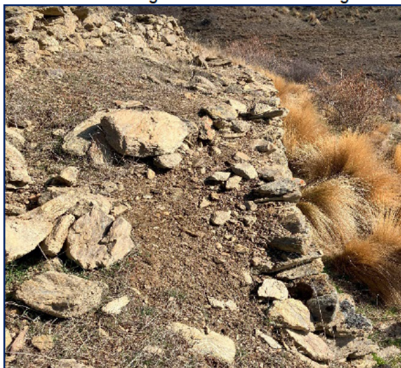
Photo C16: Rock wall above Shreks historic water dam.
