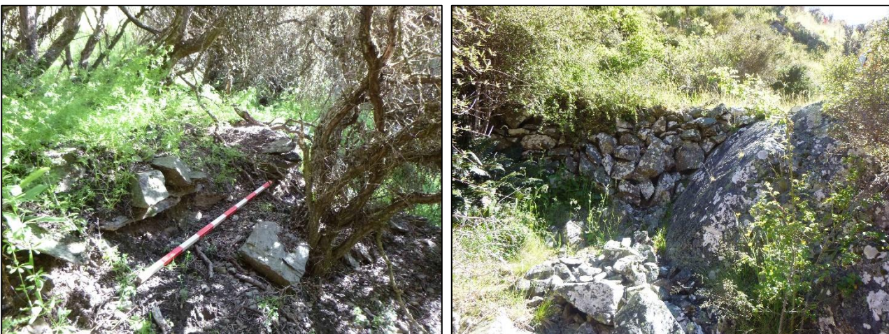
Figure 7-45 Photographs looking northwest (left) and north (right) of revetted tramway recorded as part of G41/277.
