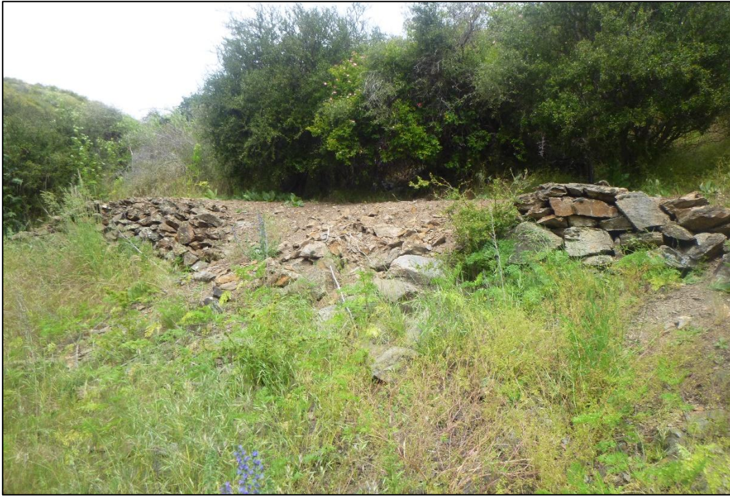
Figure 7-24 Photograph looking north at the partially collapsed stone revetment recorded as part of G41/251.
