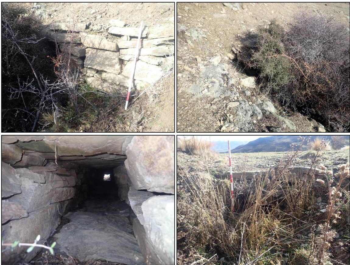
Figure 7-80. Photographs of culvert and revetment (POI 800) looking southeast at intact east end (top left), east at collapsed west end (top right), south at culvert (bottom left), and north at inlet (bottom right). Photographs taken August 2021.
