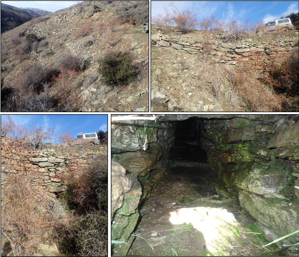
Figure 7-81. Photographs of culvert and revetment (POI 803) looking east (top left), north (top right), south at culvert (bottom left and right). Photographs taken August 2021.
