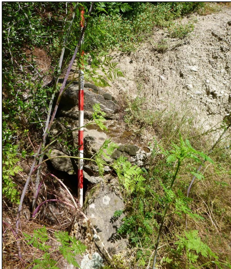
Figure 7-78. Photograph looking east at collapsed stacked schist culvert (POI 146), December 2018.
