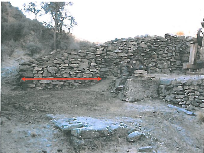
Rebuilt section of wall indicated by red arrow and borrowed pelton wheel, 30 July 2010
