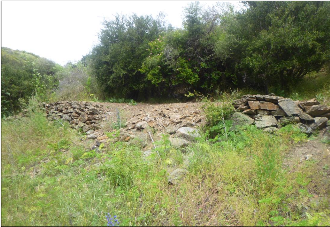
Figure 5 Photograph looking north at the partially collapsed stone revetment recorded as part of G41/251. Photograph taken by Megan Lawrence on 18/12/18.
