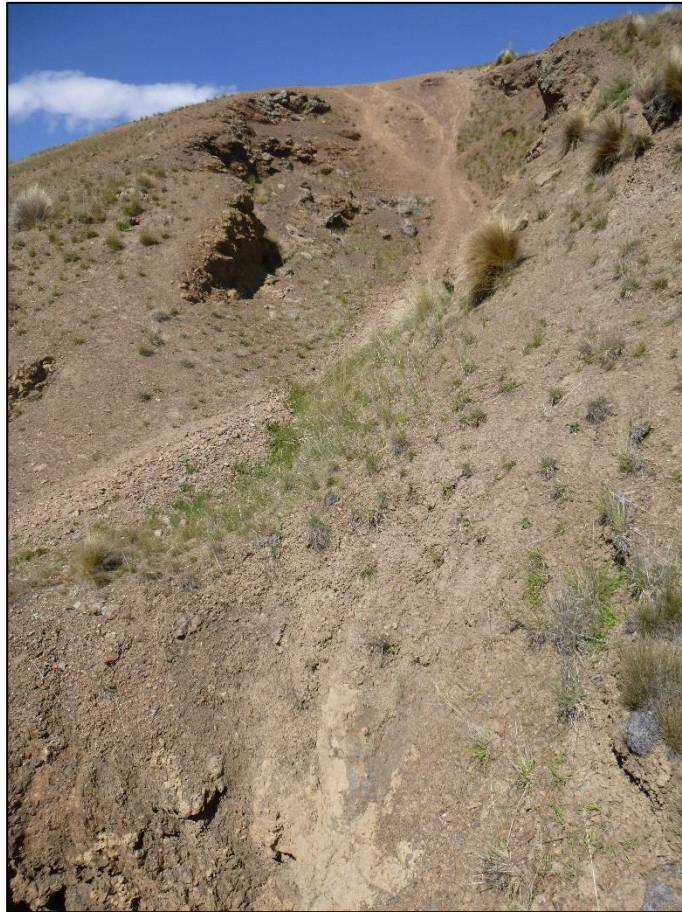
Figure 7-68. Looking southeast at G41/605, towards Thompsons Gorge Road (at top of ridge), showing motorcycle tracks, November 2017.
