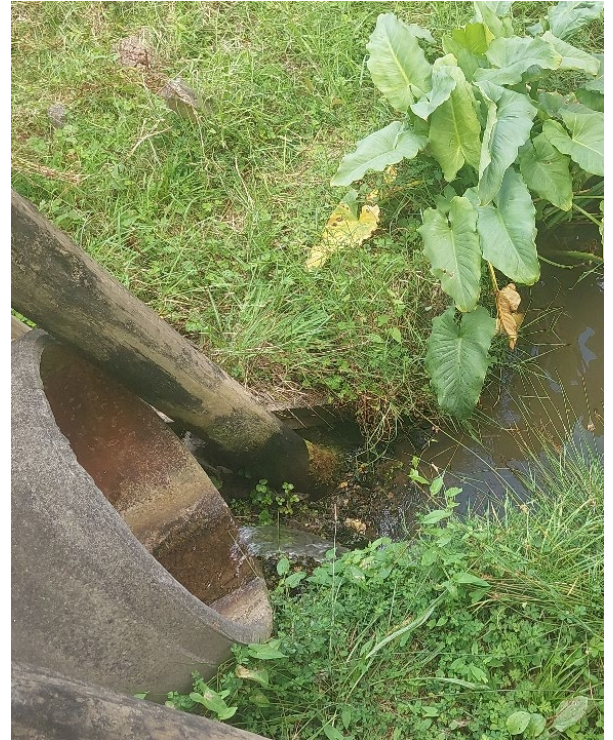
Downstream perched culvert
