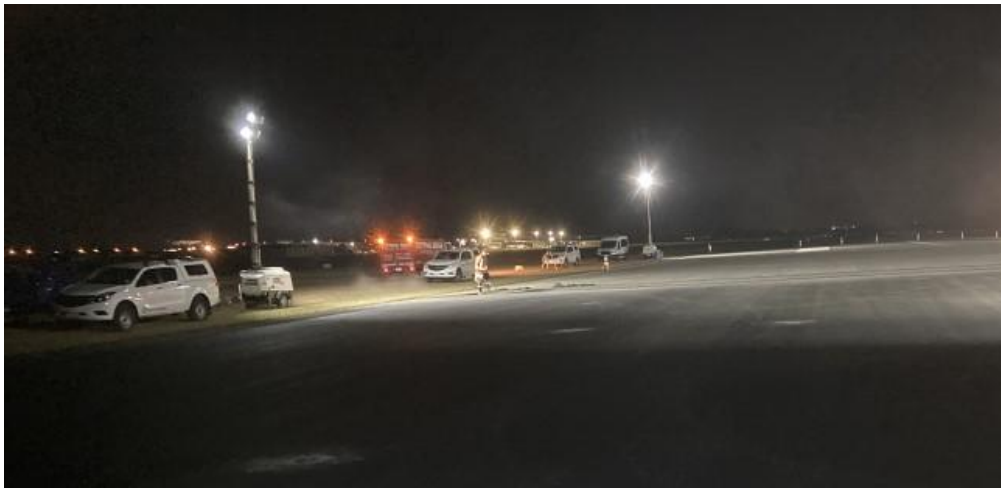
Figure 11: Typical Civil Works Mobile Lighting
