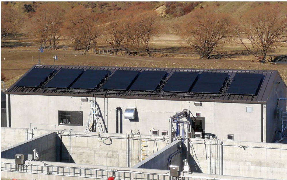
Figure 27. Solar Thermodynamic Panels at Cardrona Valley WW Treatment Plant – Alternative Energy Company
