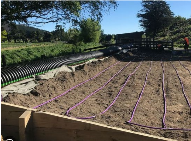
Figure 31. Purple PCDI lines and effluent arch over EcoTrench - Bray Brothers Drainage, designed by Marc Jensen
