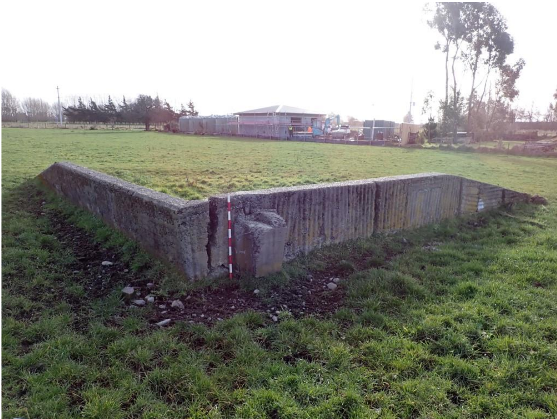
Figure 7-13. Concrete protrusion on southeast corner.
