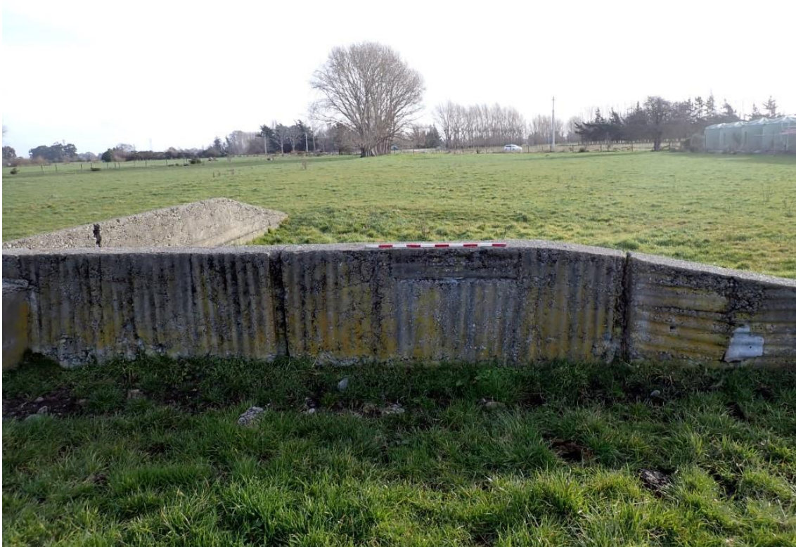
Figure 7-11. View of formwork impressions, east side.
