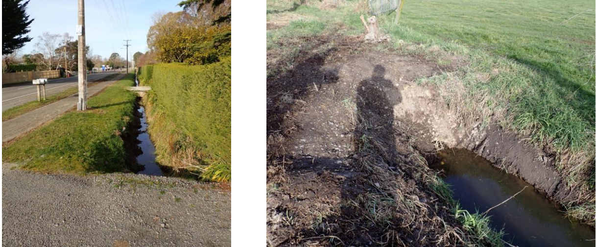
Figure 7-18. View east along the drain along the south side of Mill Road (left), and of culvert in area of embankment on Mill Road (right).
