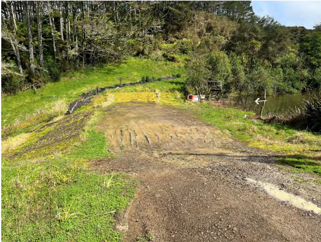
Photo 6 – Pond 5 dam crest spillway with silting and ponded water, looking west.
