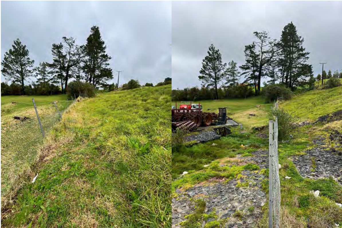
Photo 18 and 19 – Damaged fence at base of Pond 6 dam on southern side of spillway.
