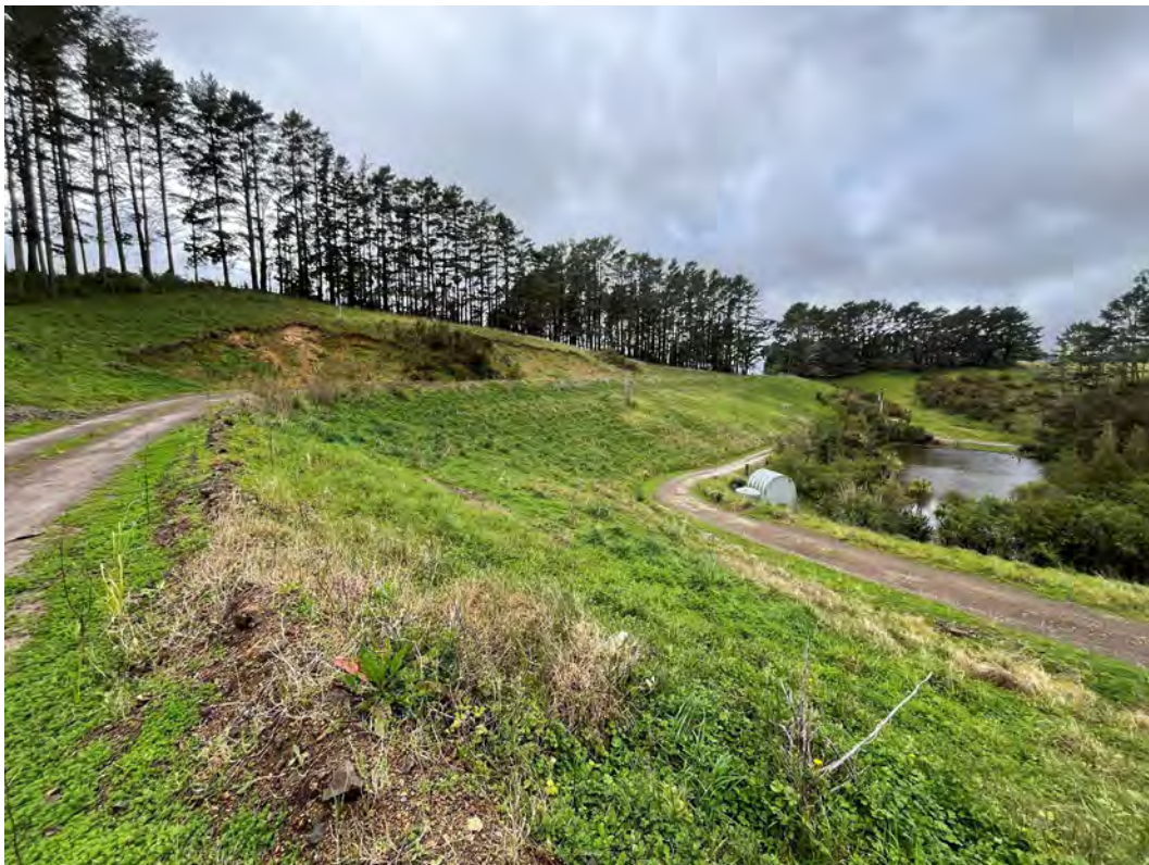
Photo 11 – Pond 5, looking southeast, cut slope instabilities visible in background.
