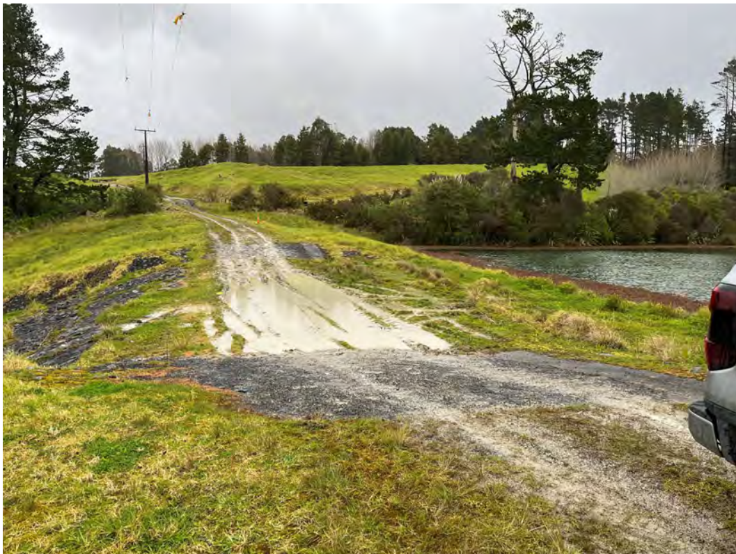
Photo 13 – Pond 6 spillway looking south, with silting and ponded water on crest.
