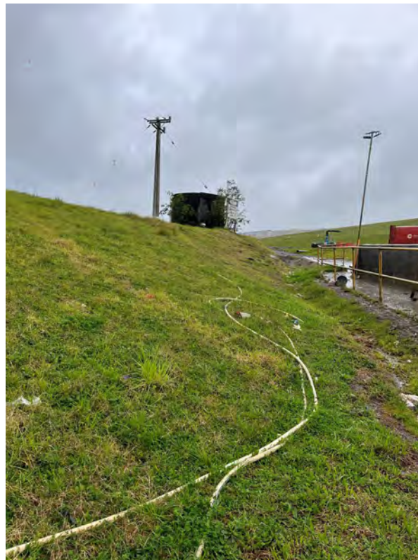
Photo 17 – Pond 6 dam with steepened slopes and concrete drainage on north side of spillway.
