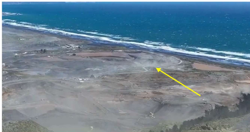
Figure 11: Visible dust from site access road on 2 March 2026
