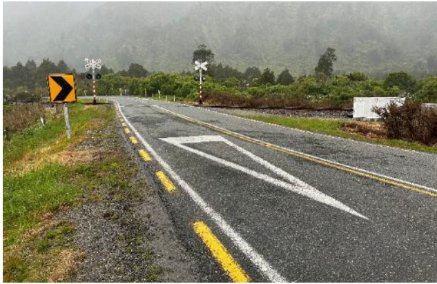
Figure 3-10: Southern approach with old give way sign still marked
