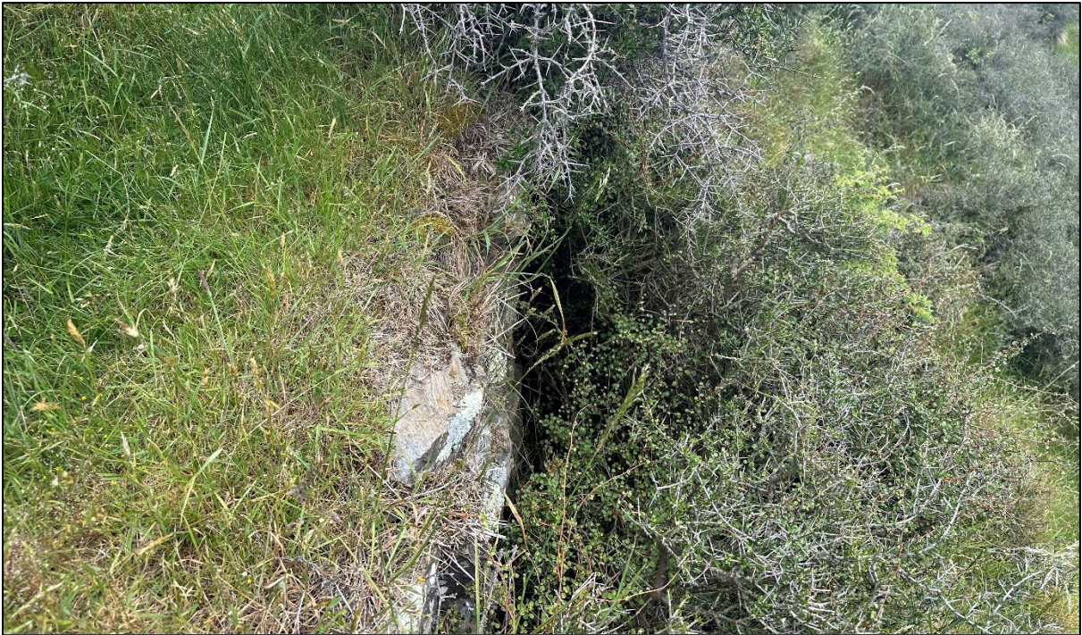
Figure 158. Heavily overgrown revetment immediately next to race (CC08), looking north.
