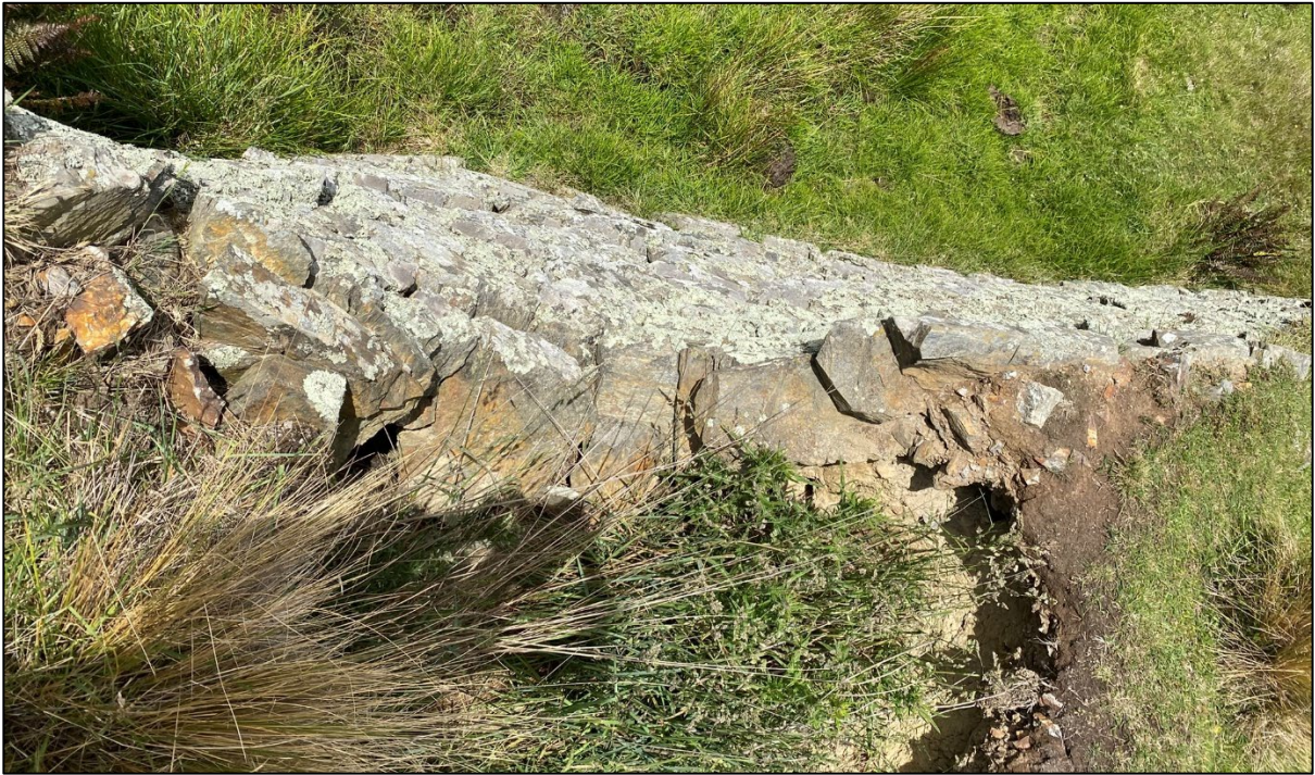
Figure 114. Condition of major revetment as shown in previous photo, looking north-east.
