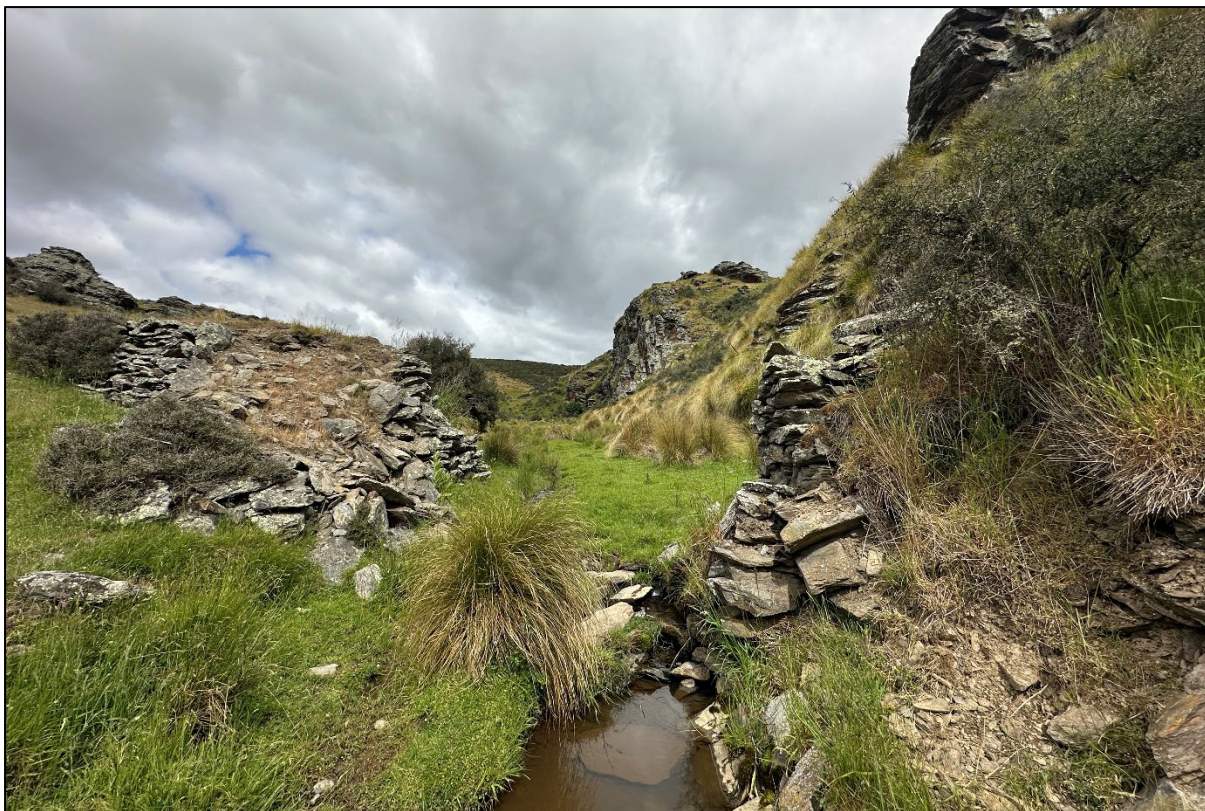
Figure 160. Breached revetment (CC09), looking west.
