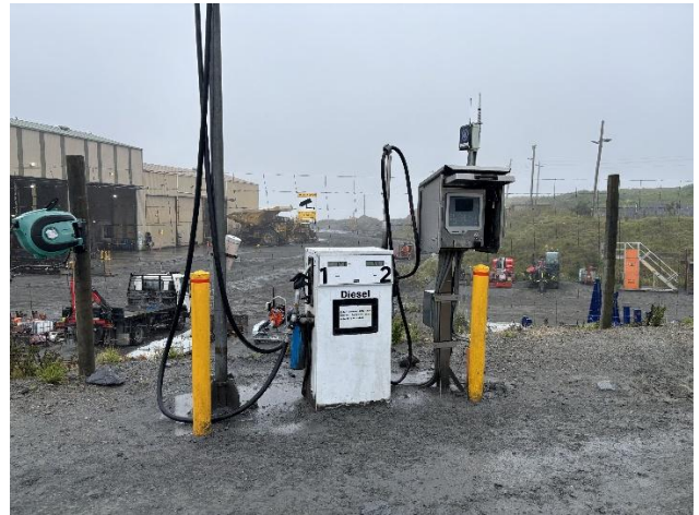
Photograph 19. Evidence of minor spills at the Vehicle Workshop Fuel Farm
