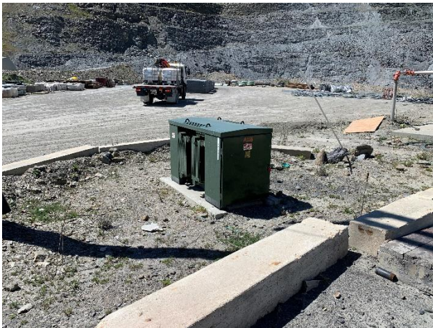
Photograph 4. Transformer at Golden Point portal
