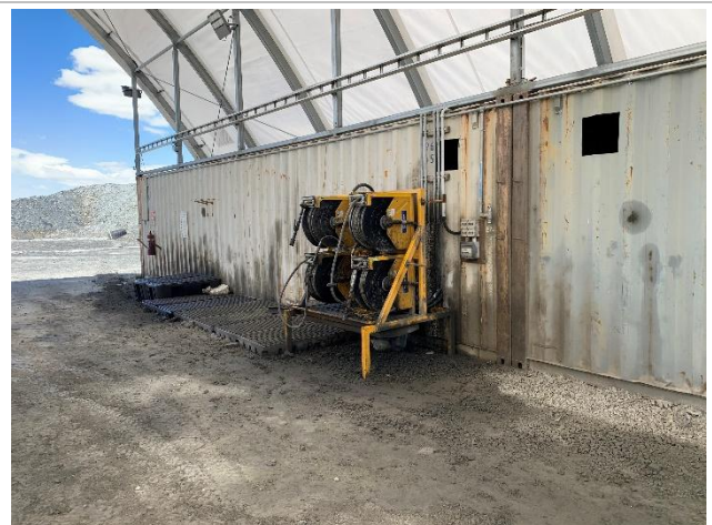
Photograph 8. Oil transfer system within former Coronation workshop
