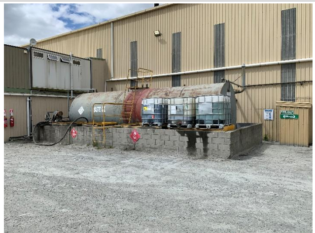
Photograph 13. Waste oil storage, banded
