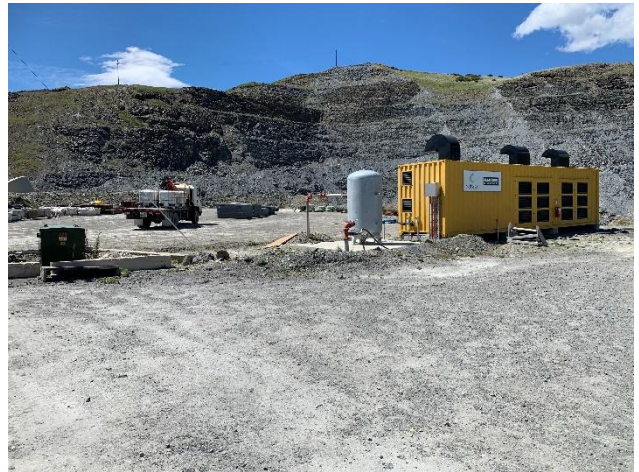
Photograph 3. Compressed air facility at Golden Point
