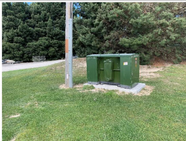
Photograph 29. Transformer next to office, typical of those on site
