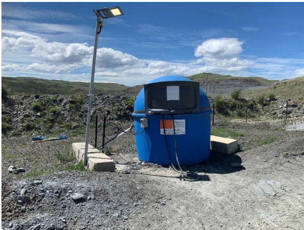
Photograph 20. AdBlue filling station, Golden Point Underground
