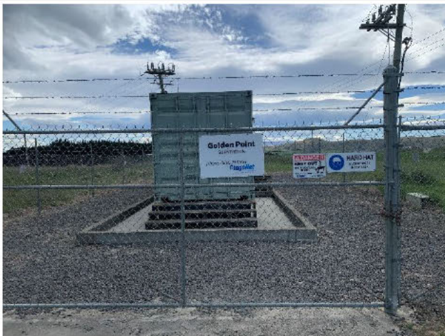
Photograph 30. Golden Point Substation
