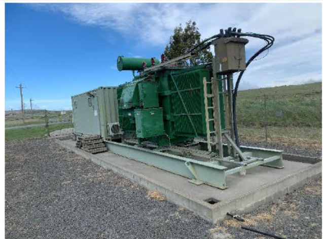
Photograph 32. Golden Point Substation
