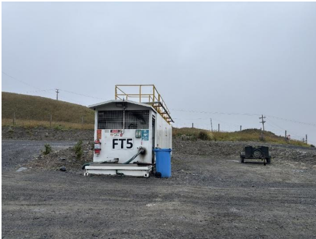
Photograph 18. Typical fuel farm set up at Vehicle Workshop
