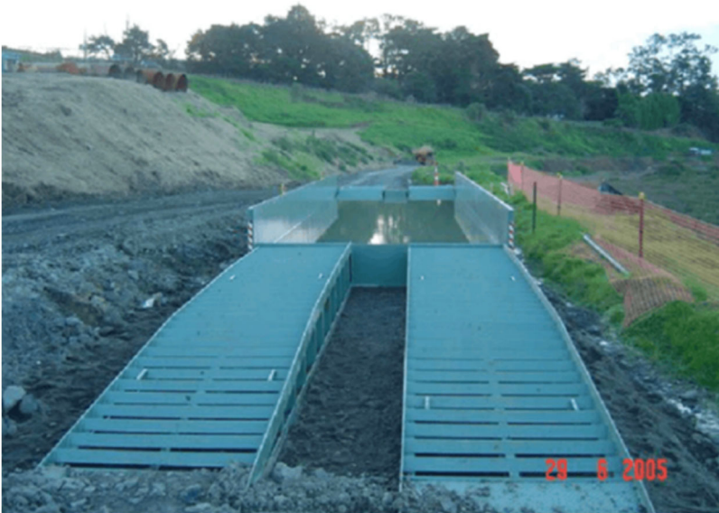
Figure 16 Example of shaker ramp provided by ECAN in the Erosion and Sediment Control Toolbox.
