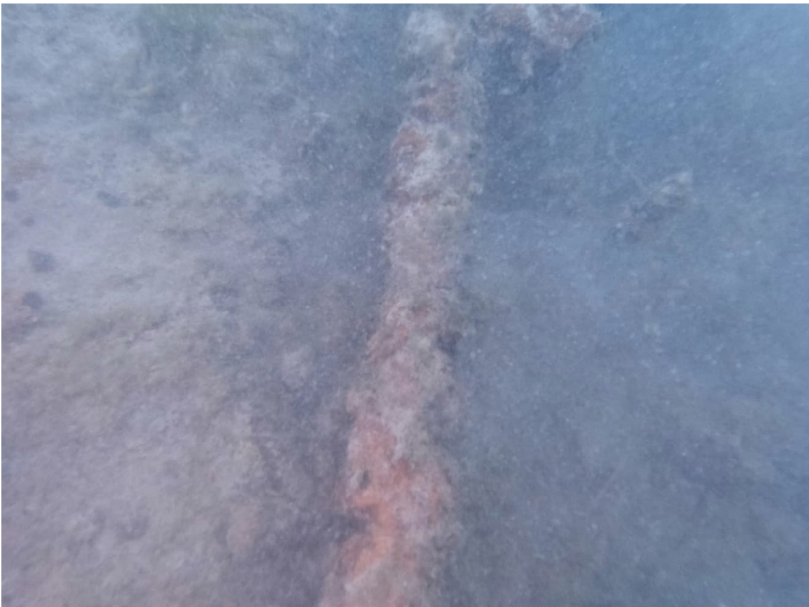
Figure 2-5. Example of exposed longitudinal reinforcement on upstream corner of weir structure.
