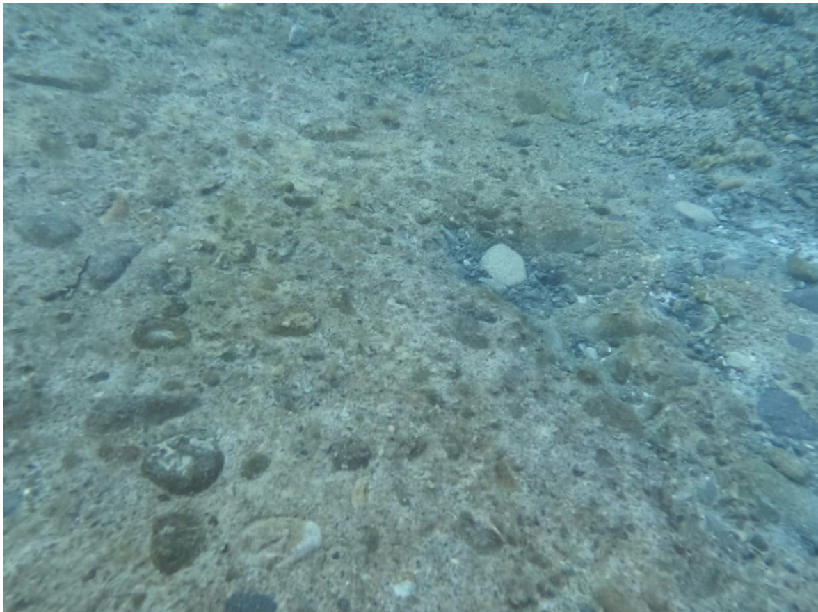
Figure 2-7. Example of exposed aggregate on the surface of the control weir.
