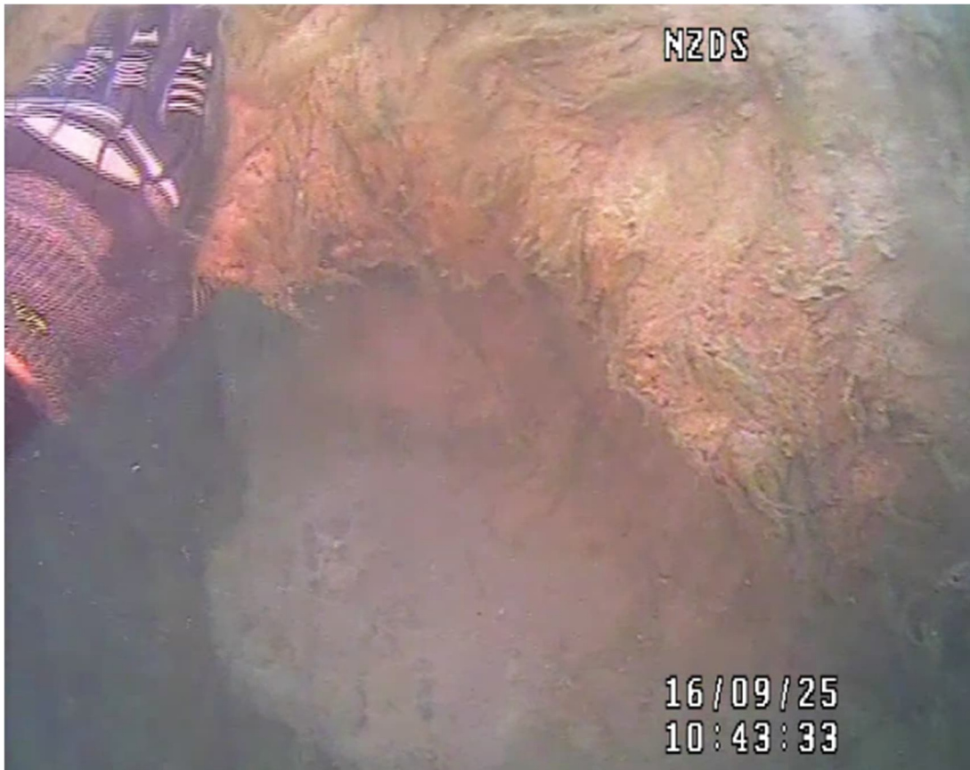
Figure 2-16. Example of downstream side of rib where rip-rap has rolled away (Rib 1).
