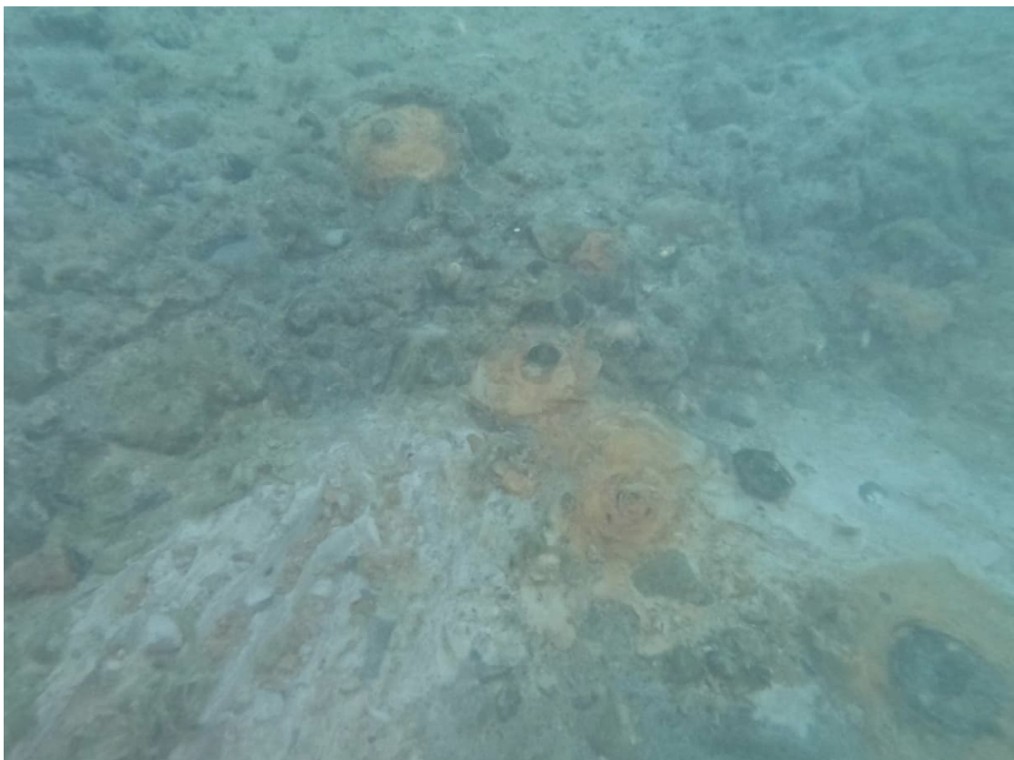
Figure 2-12. Example of exposed reinforcement on top surface of rib (Rib 1).
