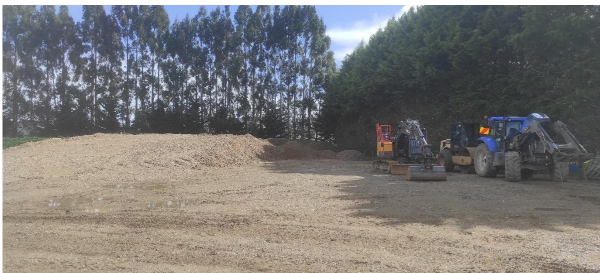
Figure 15: Recent excavation works conducted on the site to create a gravel platform (16 October 2025).
