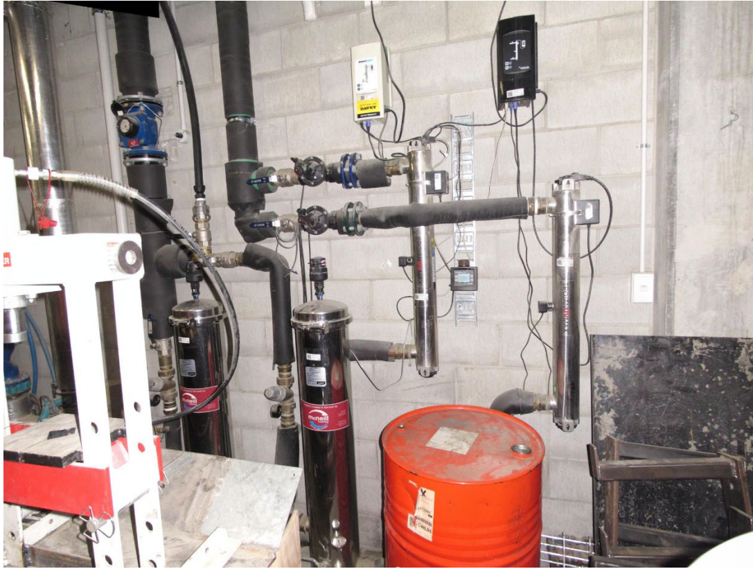
Figure 2 Existing water treatment system with two filters at lower left and dual UV disinfection
