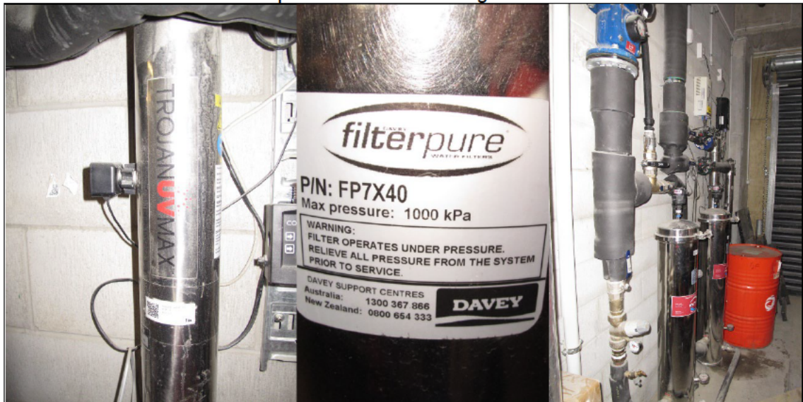
Figure 5. Elements of the existing water treatment plant with filtration and UV disinfection
