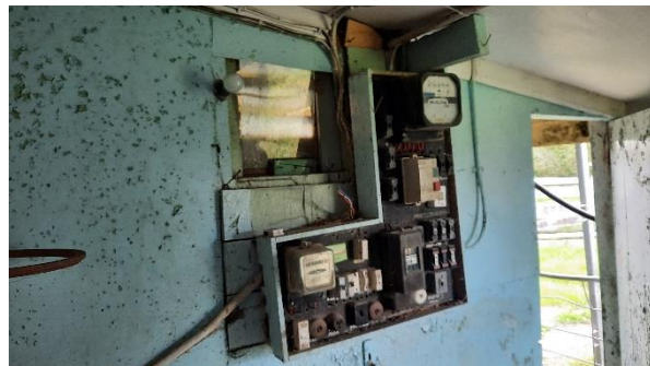
Photograph 6: Potential ACM, electrical backing board/panel
