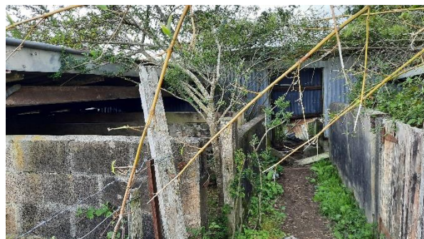
Photograph 8: Inside collapsed farm structure
