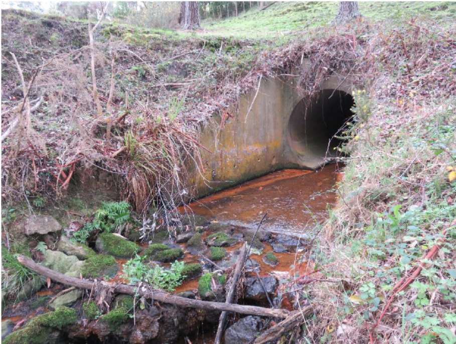
Figure 5 Eastern Culvert outlet and apron
