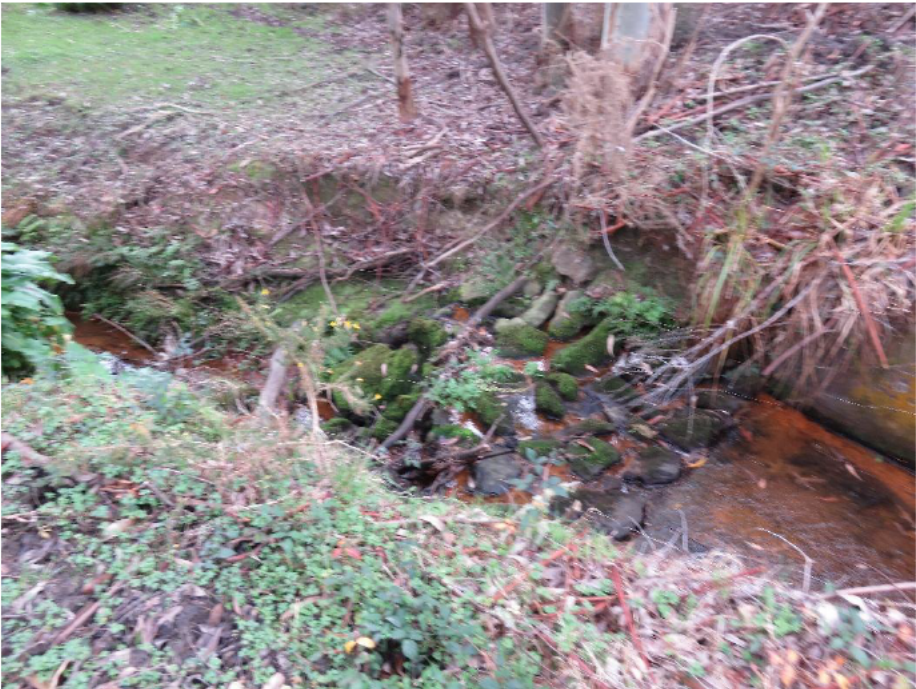
Figure 6 Eastern Culvert Outlet and Apron
