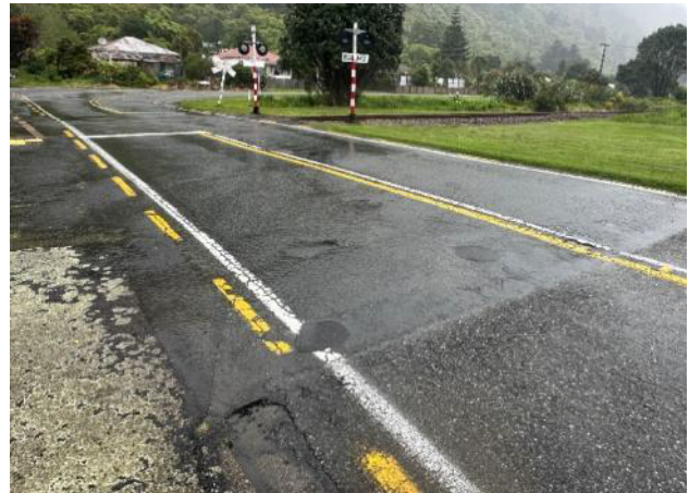
Figure 3-12: Faded line markings on the northern approach
