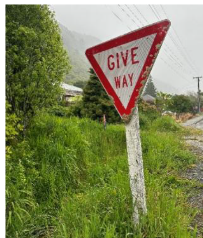
Figure 3-22: Condition of GIVE WAY sign at Back Road / SH67 intersection
