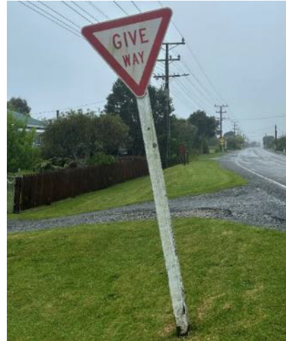
Figure 3-24: Condition of Give Way sign at Domain Road / SH67 intersection
