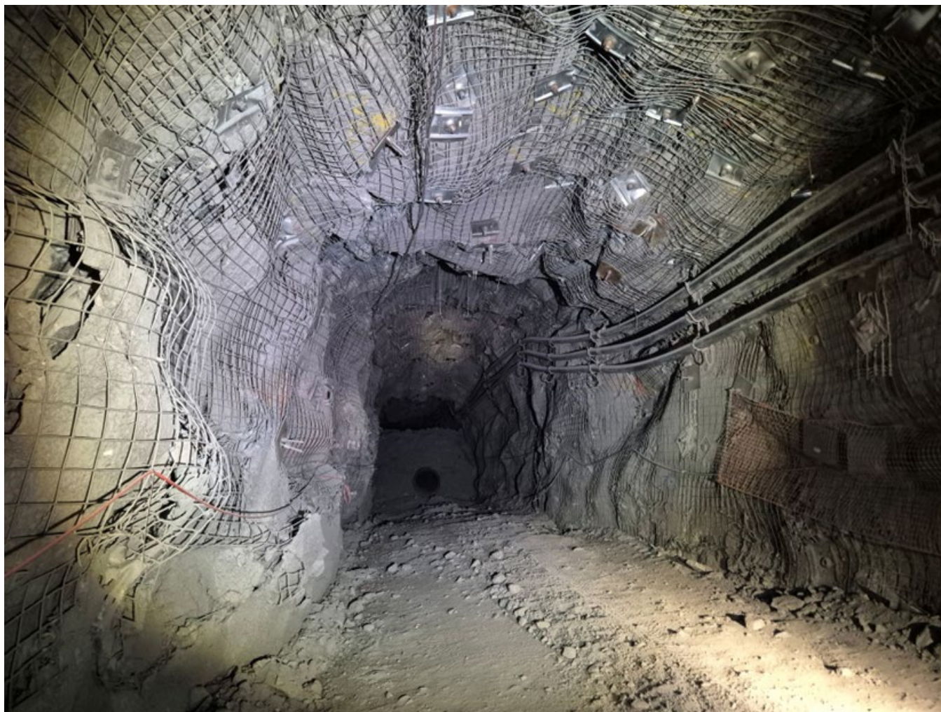
Inset 29: Photo of a development ore drive in GPUG Panel 150 showing squeezing ground.
