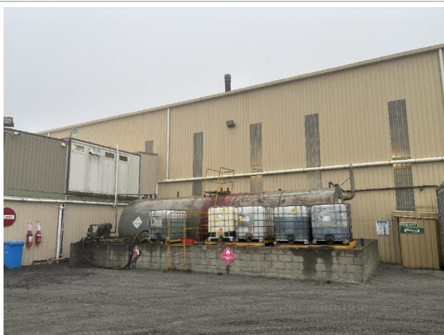
Photograph 1. Hydrocarbon storage - waste oil bund
