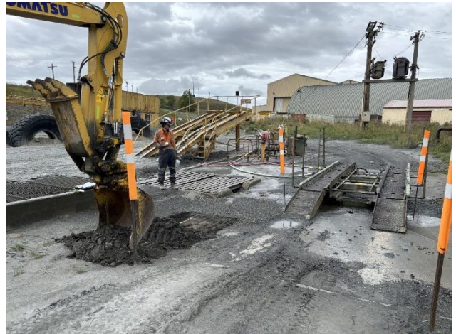
Photograph 16. Light vehicle wash bay. Sumps visible to the left and in centre of image (by person)
