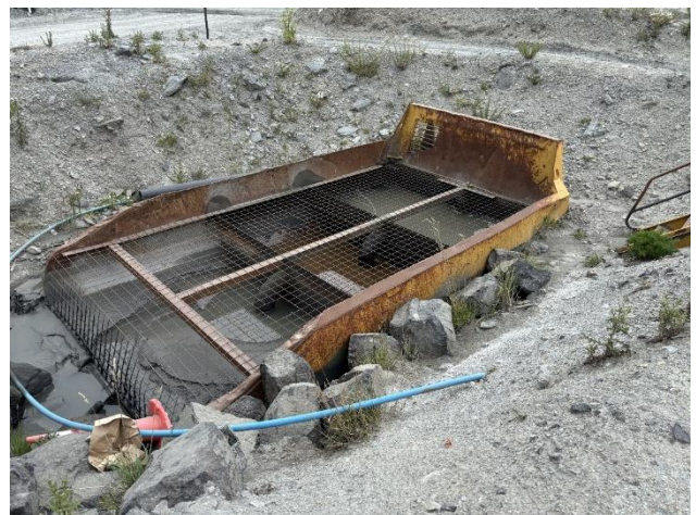
Photograph 18. Oil-water separator that services both wash bays
