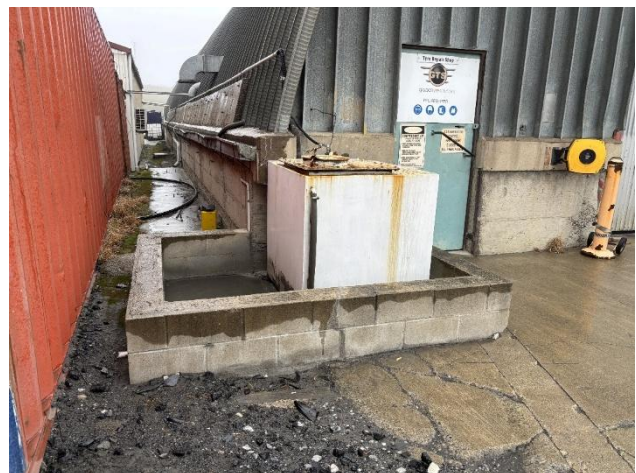
Photograph 10. Small tank and bund at tyre workshop
