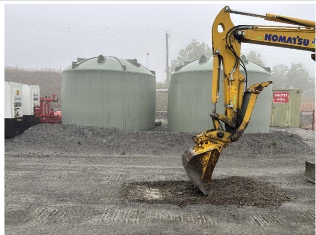
Photograph 12. Water tanks, generator storage visible to left
