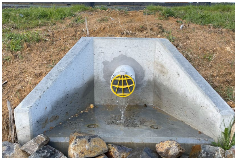
Figure 15: Backflow Device installed on Outlet Pipe.
