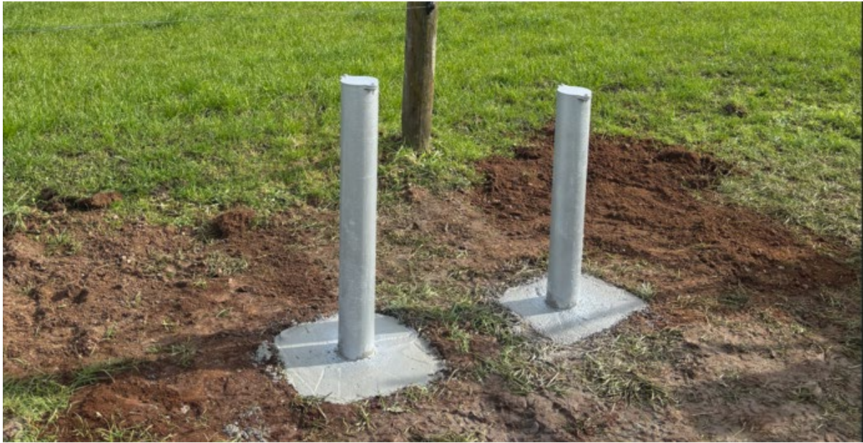
Figure 8: Twin Bore Headworks for P2S (Shallow) and P2D (Deep), Screened Above and Below the Low Permeability Aquitard Layer
