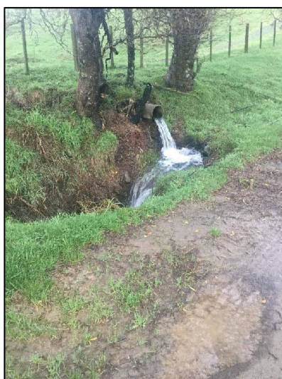
Figure 3-53: Perched Culvert on Tributary 2
