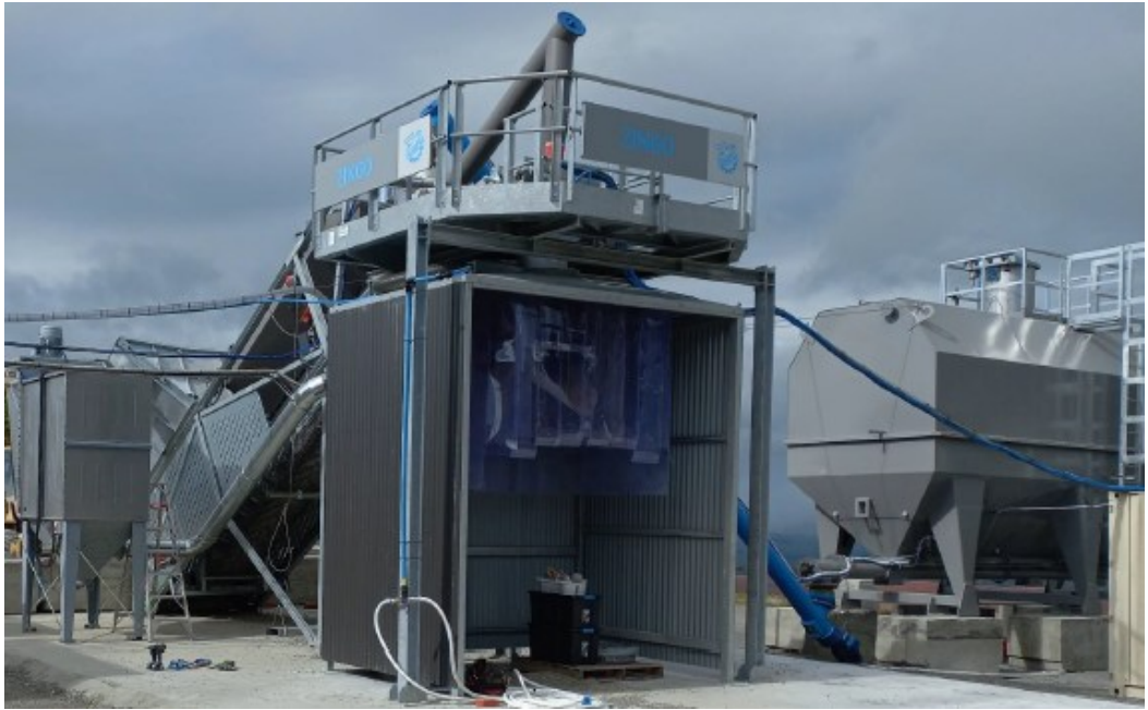
Figure 3-14: Typical Concrete Batching Plant
