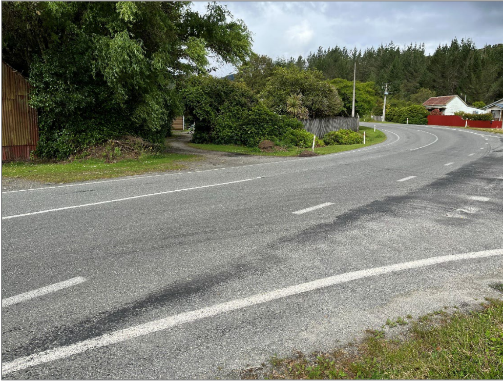
Photograph 7-2: Constrained sight lines at Soldiers Big River Road intersection
