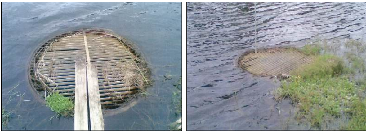
Figure 11: Pond 9 and 10 outlet structures.
