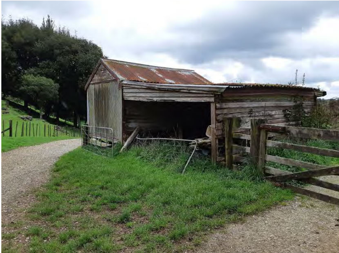
Photograph 15: View facing east of asbestos cladding on the building and roofing in the lean-to at Building 3.
