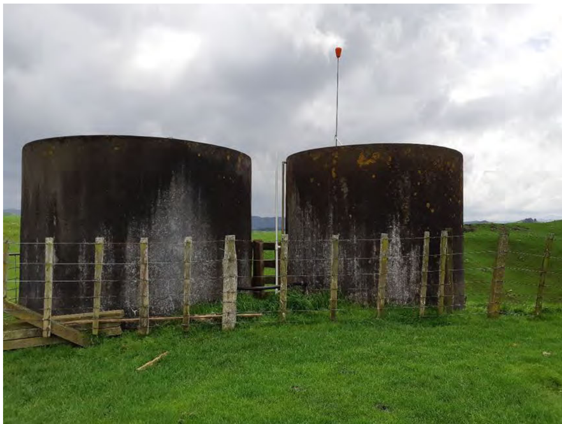
Photograph 5: View facing north of water tanks in the north-eastern portion of the site.
