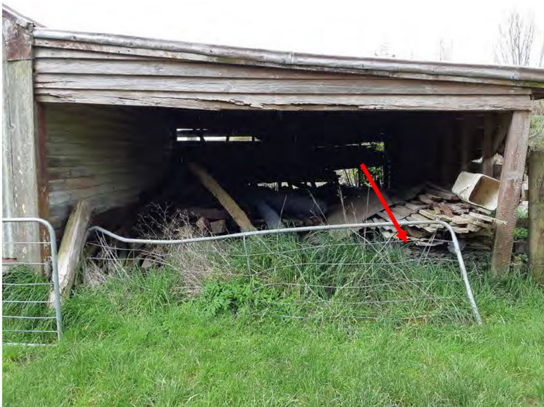
Photograph 16: View of asbestos cement sheet being stored in the lean-to at Building 3.
