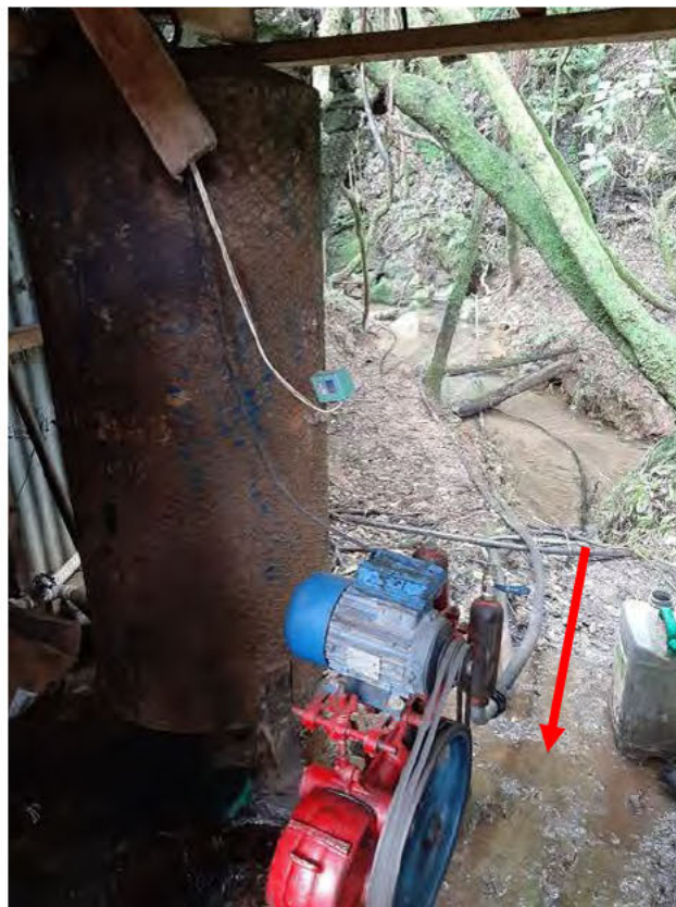
Photograph 18: View of the pump within Building 4; a small stream is visible beyond the building. Minor motor oil spill identified by the arrow.
