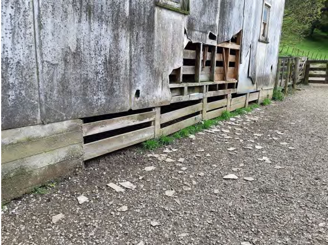
Photograph 13: View of broken asbestos containing cement sheet on the southern exterior wall of Building 2.
