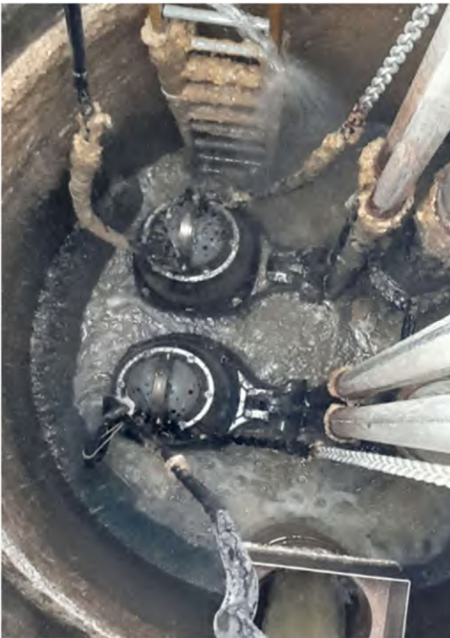
Figure5: Pumpsets located in wetwell.
