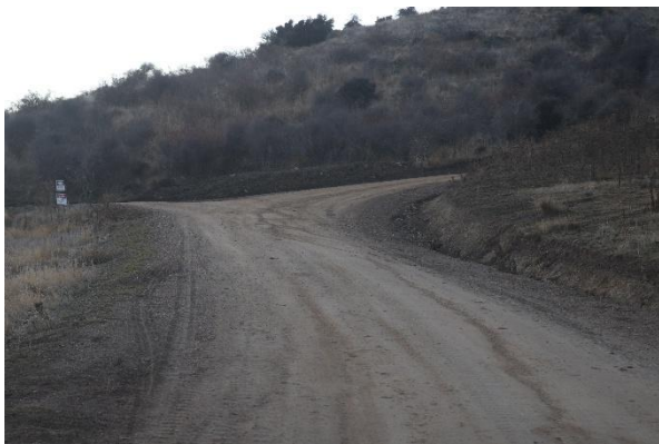
Figure 5: Tight alignment with surface rilling 1
