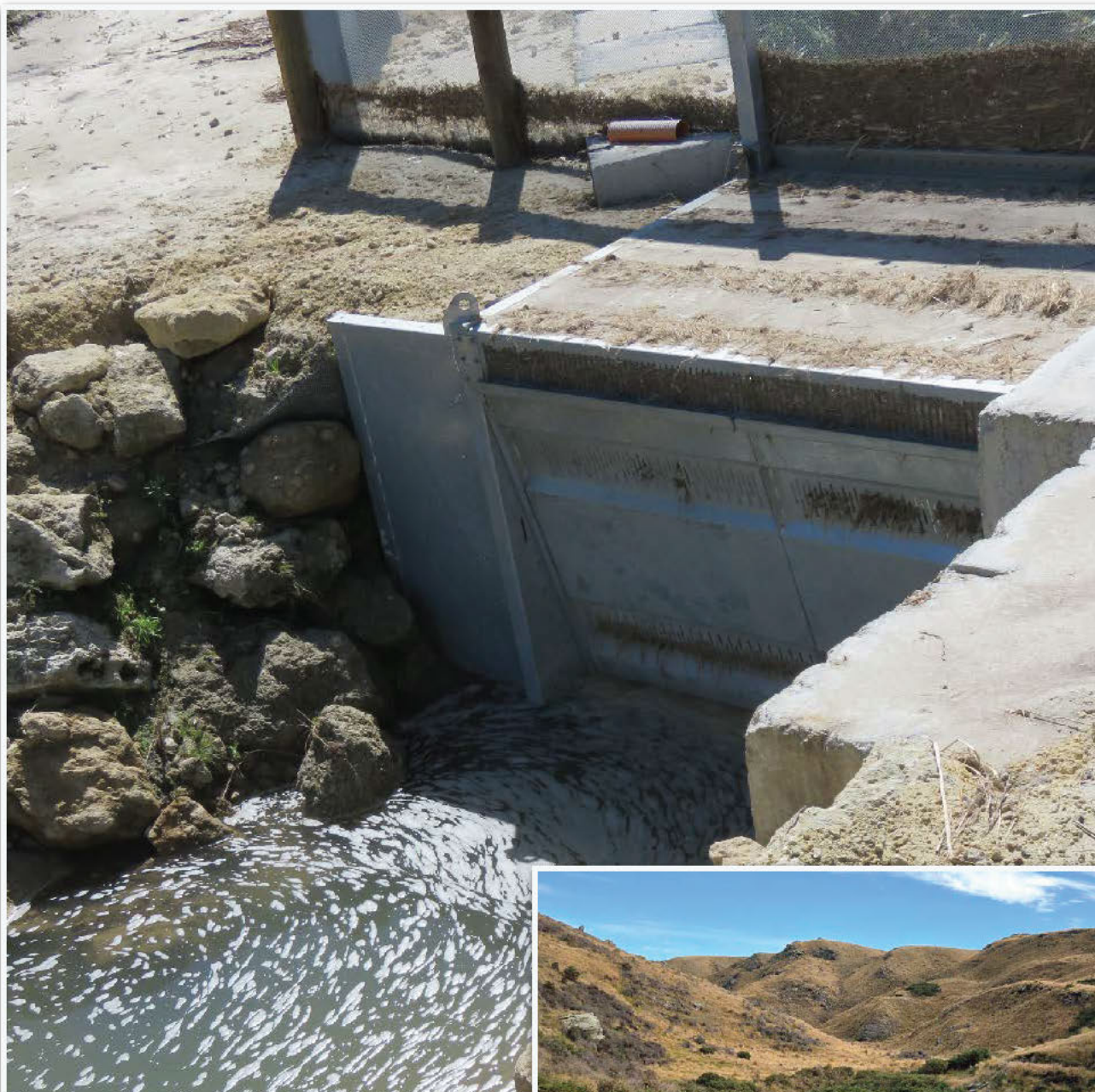
Fig. 8a. Example of a large inflow culvert, mounted on a concrete foundation, appropriate for the site.
