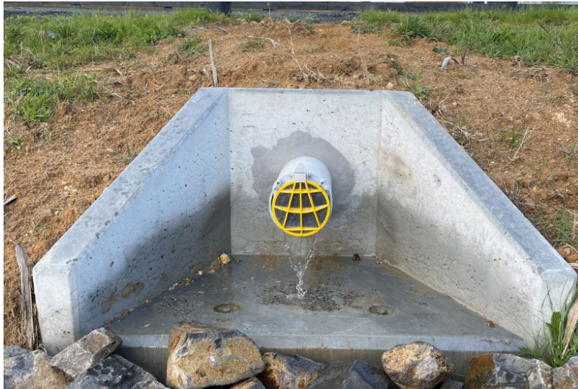
Figure 16: Backflow Device installed on Outlet Pipe.
