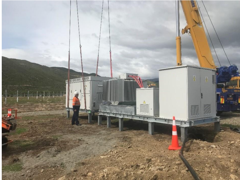
Figure 8- MV Transformer Station
