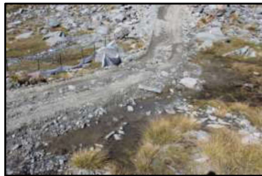
Figure 82. Same area after trench dug, pipeline laid and buried. To orient oneself note large rock upper centre left. Lower centre in Fig. 81.
