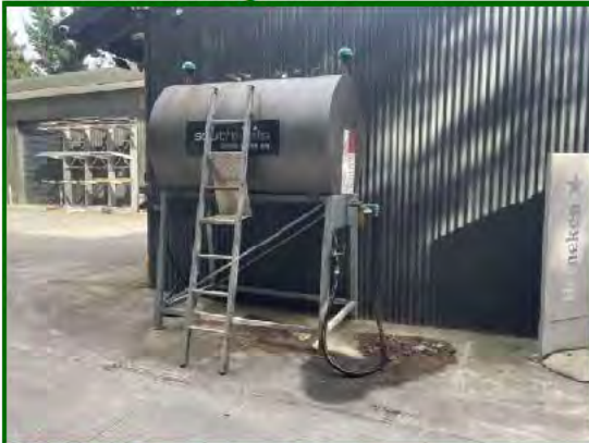
Photo 7 – AST and minor staining
