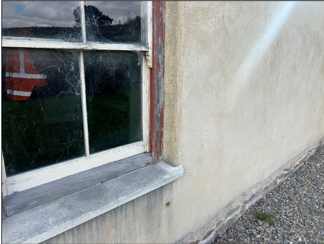
Photo 3 Bare timber to one of the windows (east elevation).
