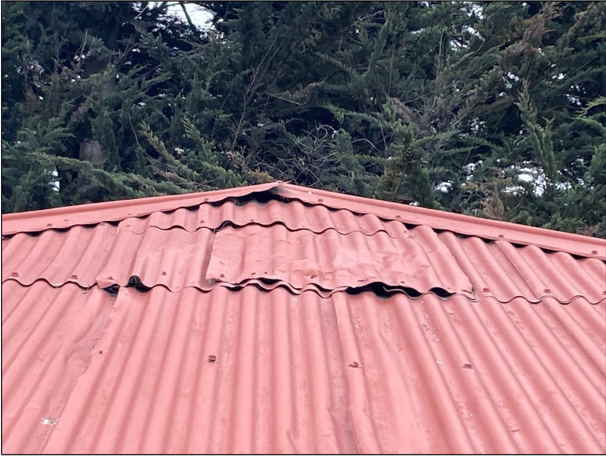
Photo 1 Loose ridge flashing & roofing.
