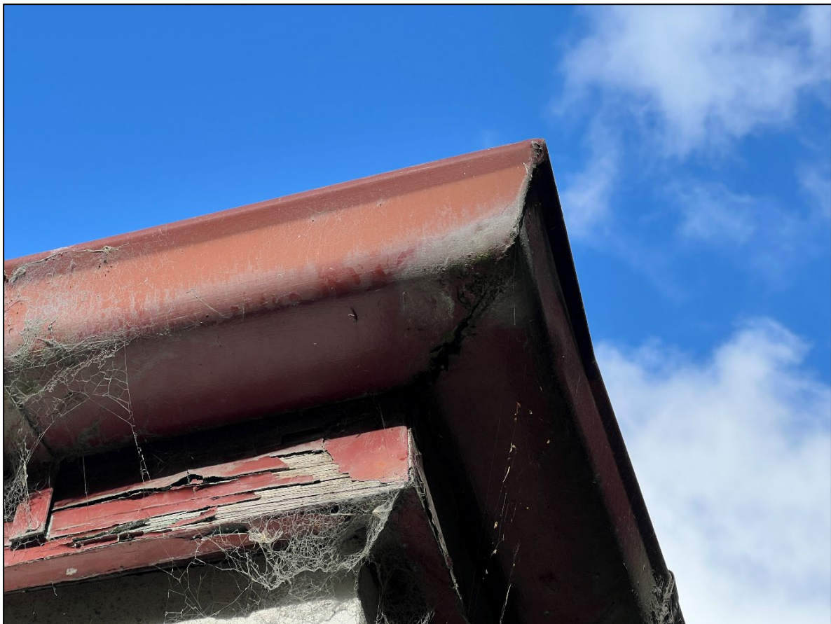
Photo 4 Leaking joints to guttering; decaying fascia board
