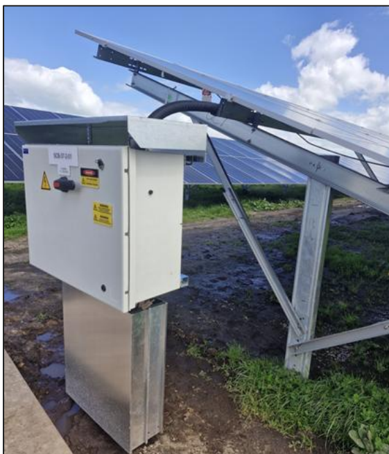
Figure 12: Example String Combiner Box
