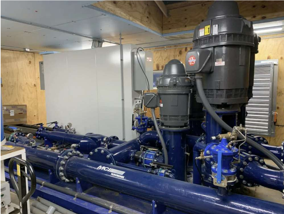
Figure 27: Large skid mounted multistage snow making pumps within a timber building.
