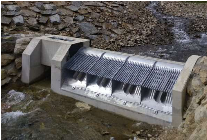
Figure 23: Coanda Wier Intake – JX Filtration
