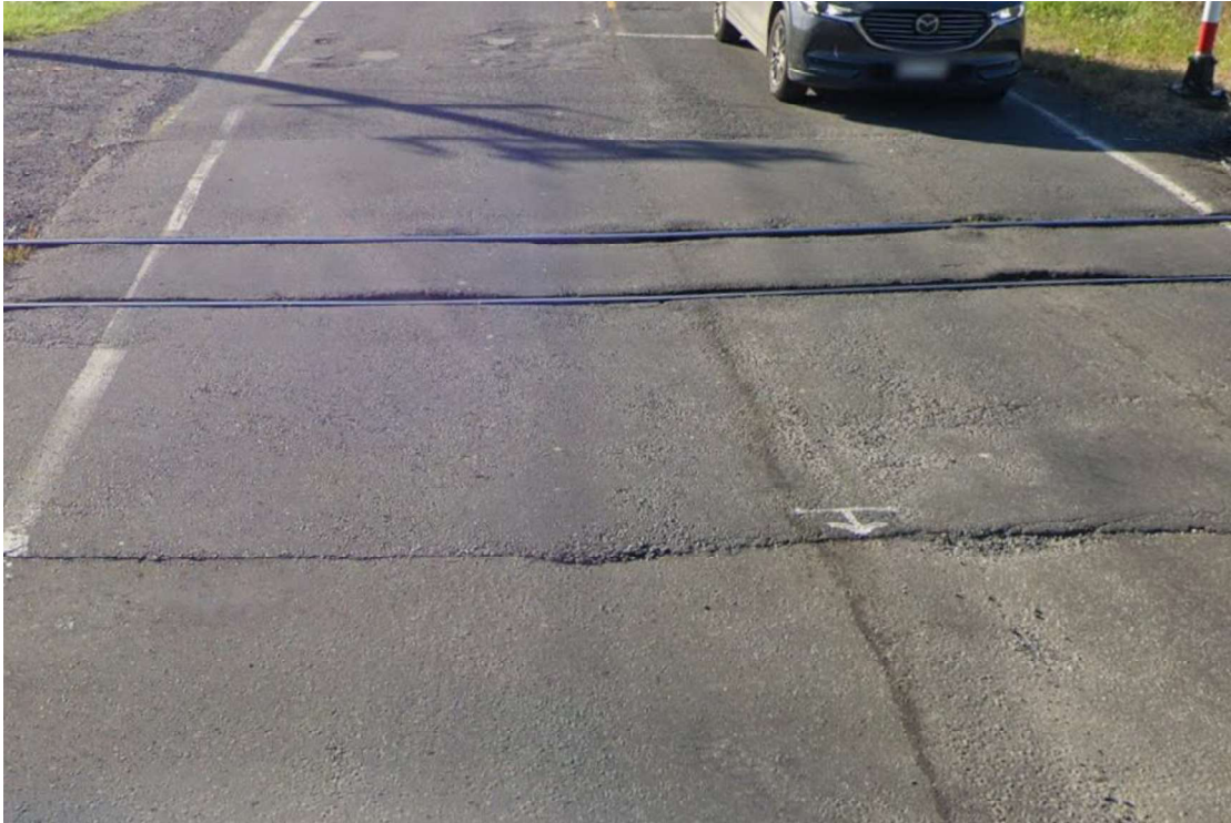
Figure 5-6: Level crossing surface flange gaps (source: Google Maps)
