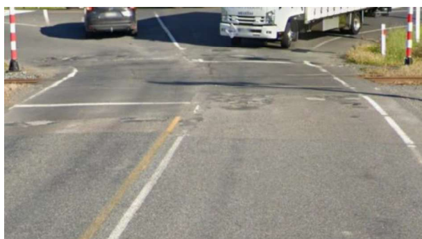
Figure 5-4: Eastern approach surface rutting (source: Google Maps)
