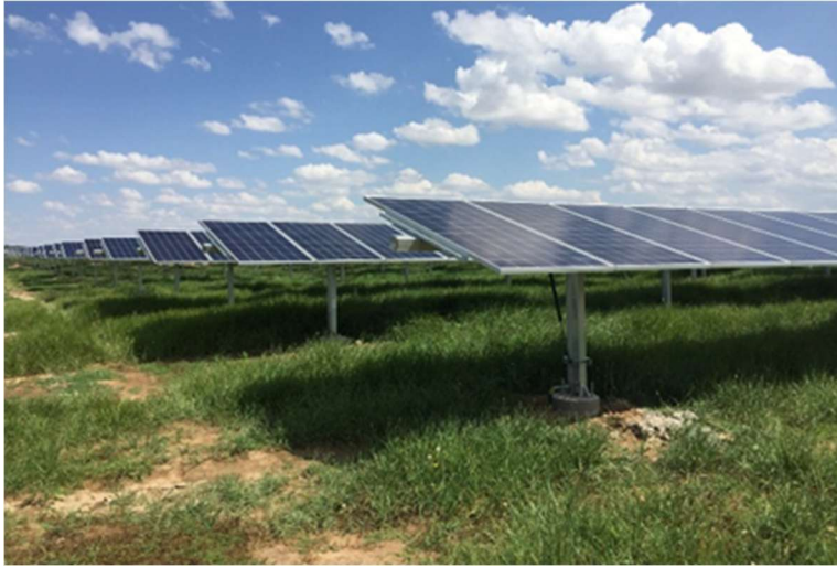
Single-axis solar tracking panels
