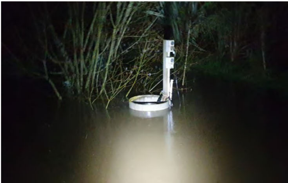
SUMP ALMOST SUBMERGED DUE TO FLOODING FROM OHOKA SOUTH BRANCH (WATER DEPTH > 750mm)
