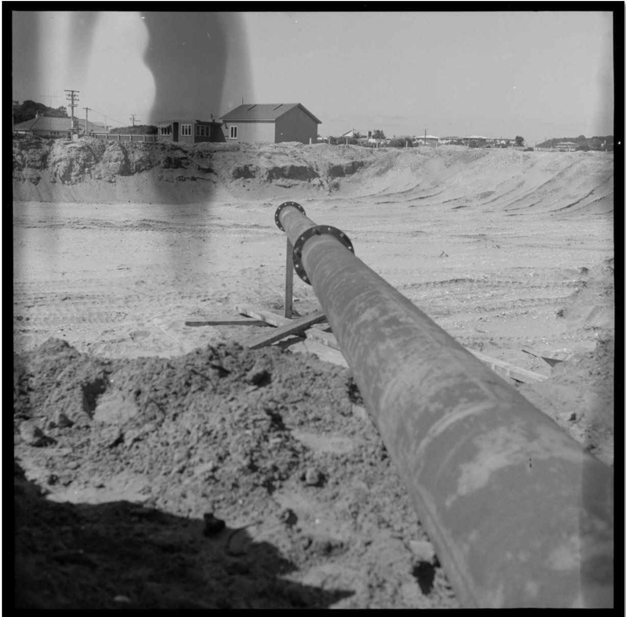
Figure 30: Dredging pipeline for Mount Maunganui wharf extension; 1967. Tauranga City Libraries, photo gca-14671.
