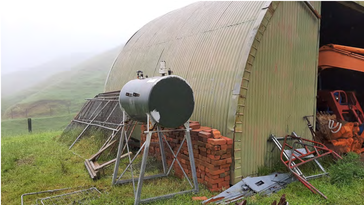
Photograph 9: AST located at the storage shed in the central portion of the site. No staining on the ground beneath the AST is noted, and the AST appears to be in good condition with no leaks visible. No labels are visible on the AST.
