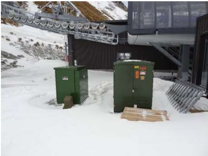
Photo 2 – Typical RMU (left) and Kiosk Transformer (right)
