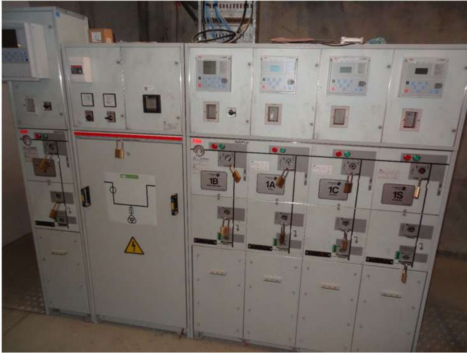
Photo 1 - Existing 11kV Switchboard
