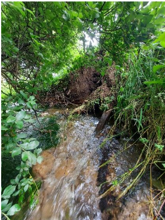
Photo 11: Active erosion of channel banks downstream of Pōtea Spring
